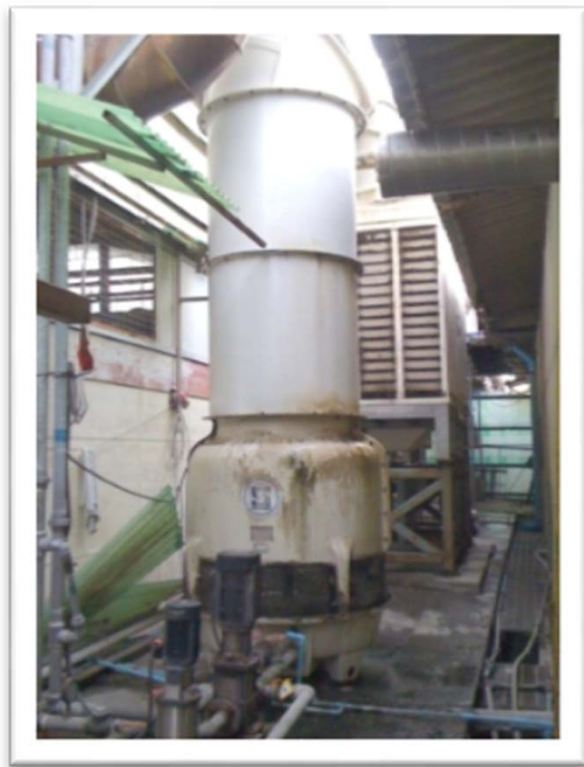
Open circuit cooling tower 125 TR + 50 TR
