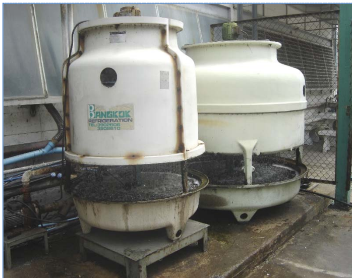
Open circuit cooling tower 40 TR + 15 TR
